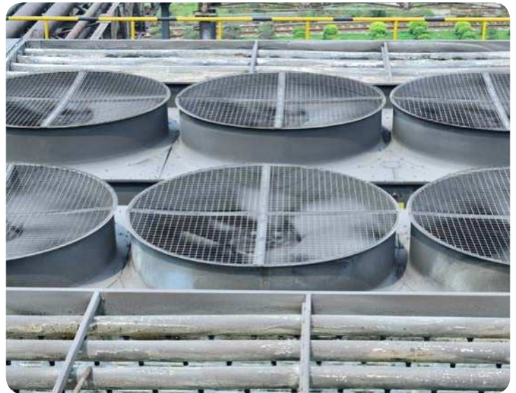
Cooling tower fans are applied throughout the downstream industry and pose specific maintenance challenges for which SKF has developed a broad range of solutions.
